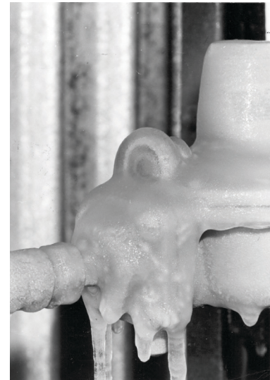
VENTS ON HORIZONTALLY MOUNTED REGULATORS BECAME QUICKLY PLUGGED DURING FISHER'S TESTS.
