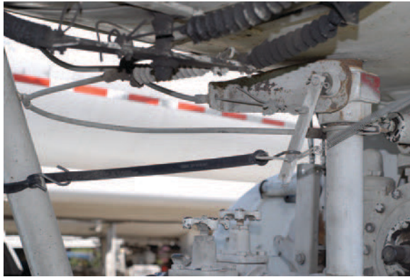
THE CABLE SHOULD BE AT A RIGHT ANGLE TO THE OPERATING LEVER AT THE MID-TRAVEL POSITION.
